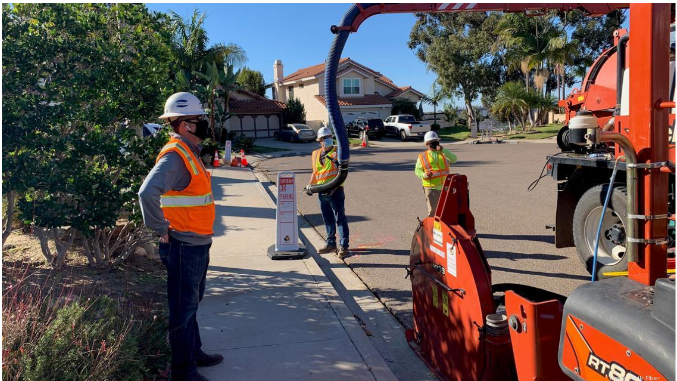
A Netly Fiber crew lays high-speed fiber cable along a residential street near San Diego.
